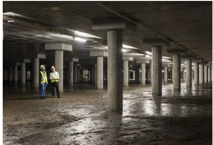
Hong Kong's Happy Valley Underground Stormwater Storage Scheme uses a large underground tank to store the surge of stormwater runoff which reduces downstream flooding risks during severe rainfall events. Photo: © Black & Veatch
